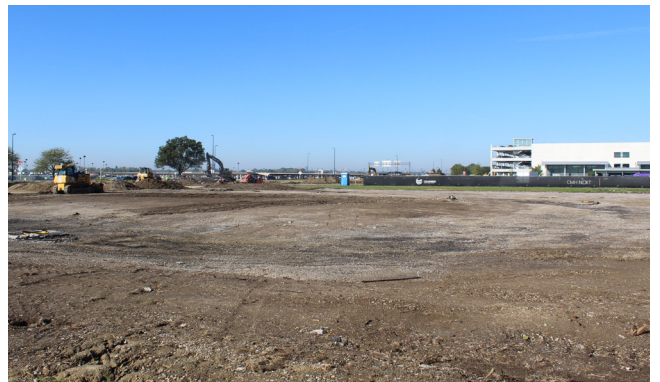
Clearing the way for what's next: the demolition of McDonald's was completed in September.
